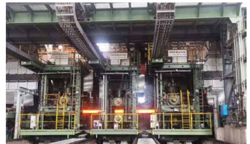
— The centerpiece of the plant: the CCS® (Compact Cartridge Stand) tandem rolling mill unit with hydraulic adjustment system and fully automatic quick program-change function.
