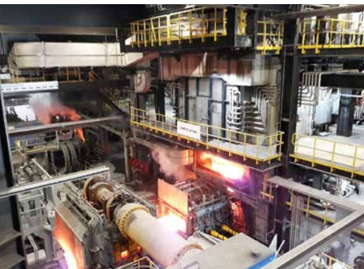
With a maximum strip width of 1,930 millimeters, it is one of the widest kinds of its kind in the world: the No. 2 CSP® continuous caster with pendulum shear at Big River Steel.
