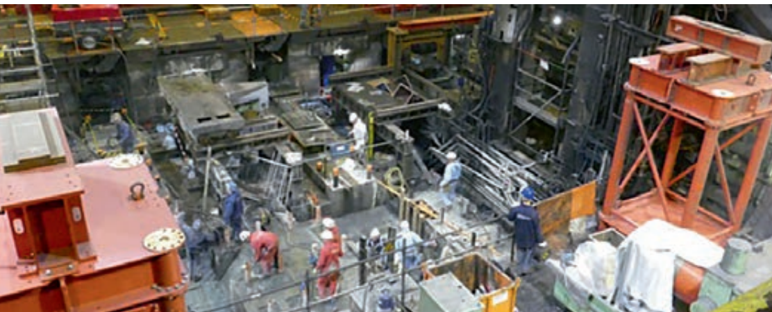
Finishing mill in the area of the rolling stands F1 and F2. Second week of second shutdown: installation of the new stands.
