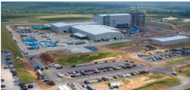
Aurubis, USA – the first multimetal recycling plant in the US
