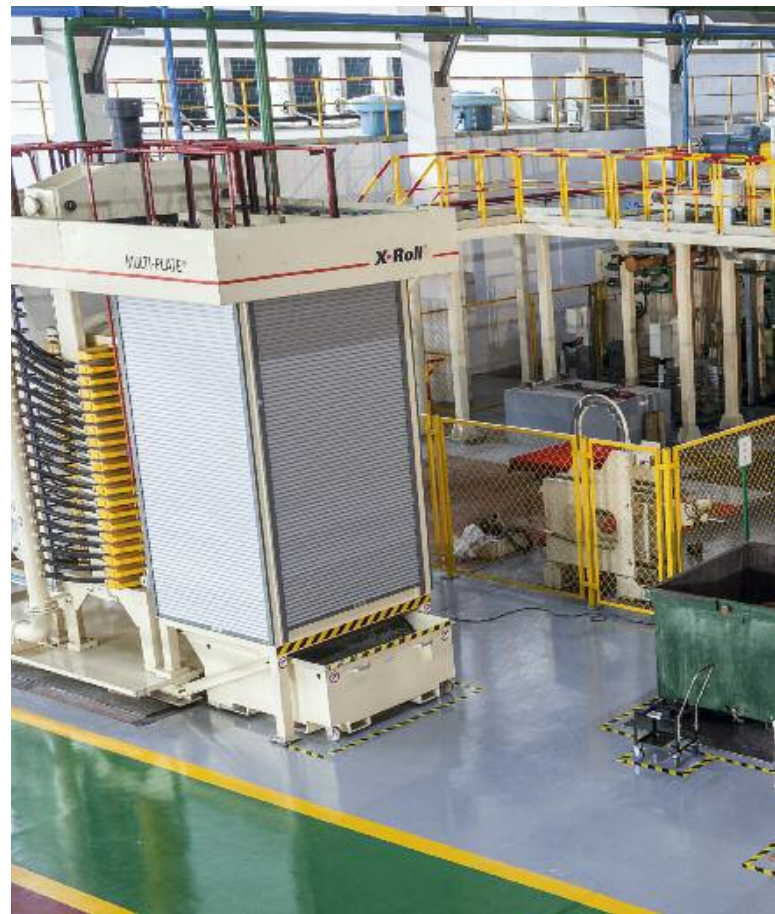
The auxiliary equipment of the thin strip cold rolling mill operated by Ningbo Xingye.
