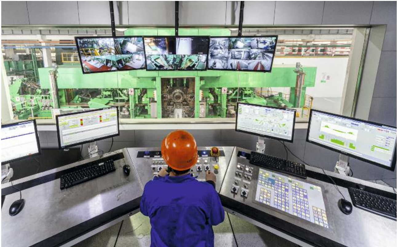
State-of-the-art control centers are hubs where all the relevant information about the fully automated rolling process comes together and is visualized.
